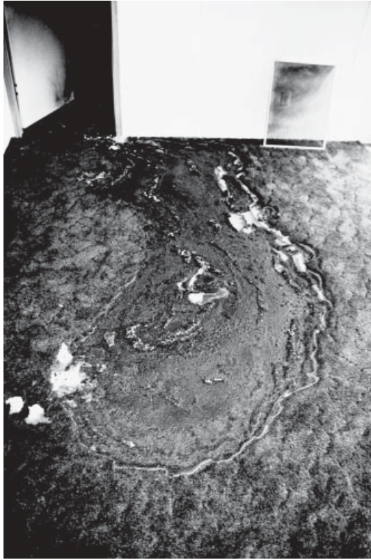
Figure 3.1 “Obvious pour pattern.” The only surface that was burned in this mobile home was the floor. There were no furnishings in the house. The carpet was tested and found to be positive for the presence of a medium petroleum distillate such as mineral spirits or charcoal lighter fluid. This is a unique case where visual observation alone can lead to valid conclusions about what caused the pattern. ( See insert for color representation. )
